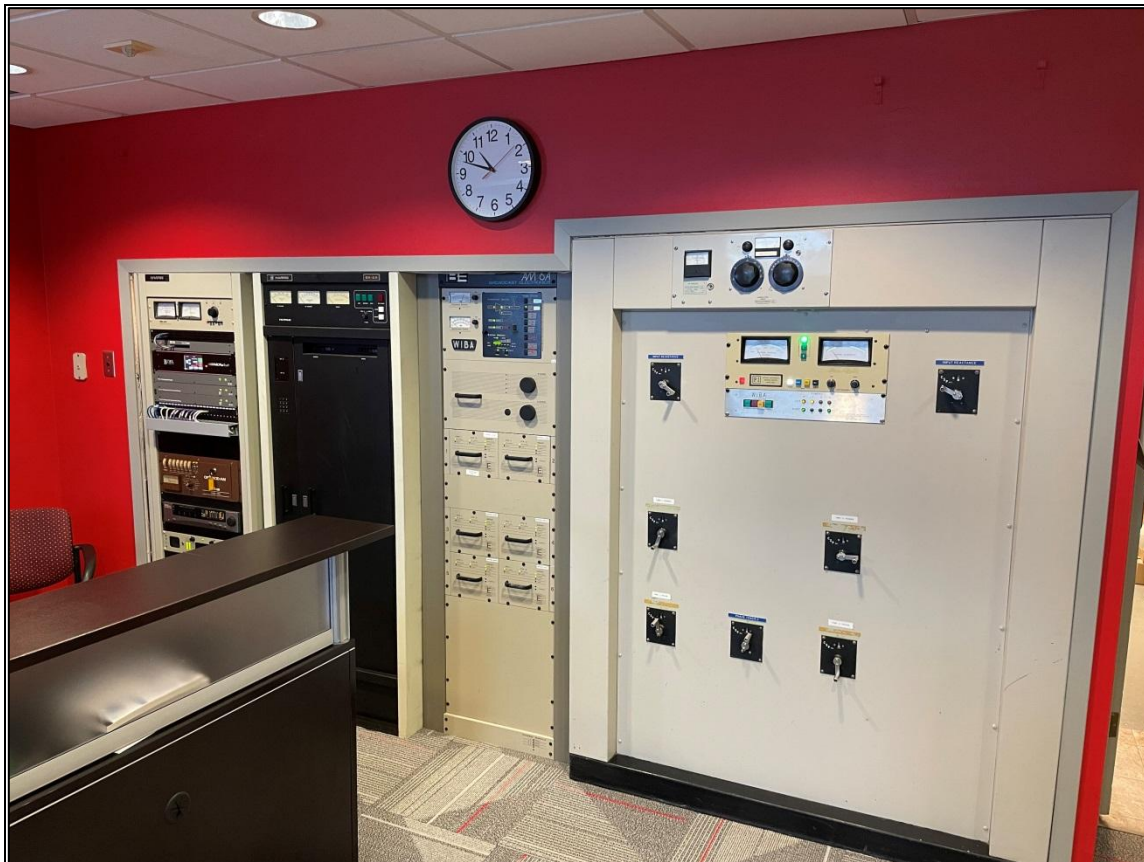
Lobby view with the transmitters.
