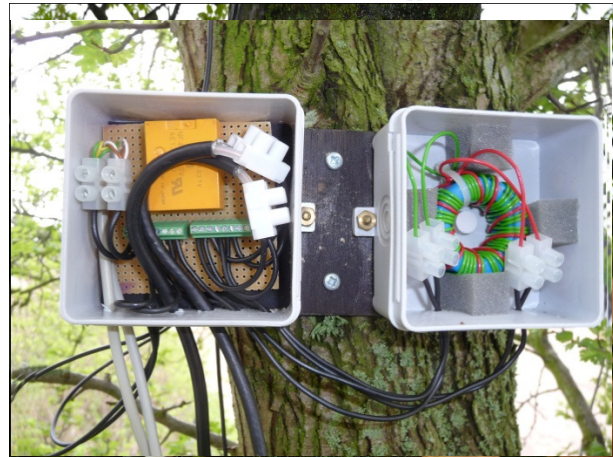
Interior view of the 10x10 cm boxes on the right antenna side. The left box contain the relay and termination blocks on the circuit board, the right box contain the balun.
